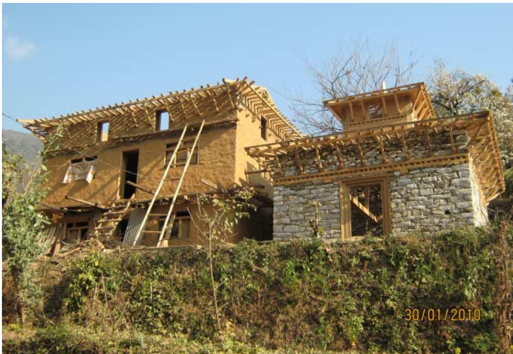
FIGURE 1. Bhume temple renovation underway in 2010, funded by JANSEEP. Photo by Bir Bahadur Thami
